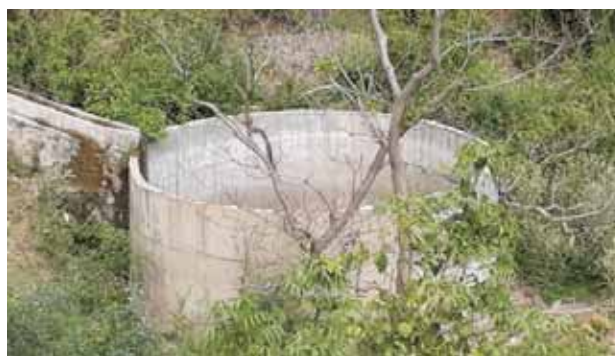
Water storage tank for irrigation
